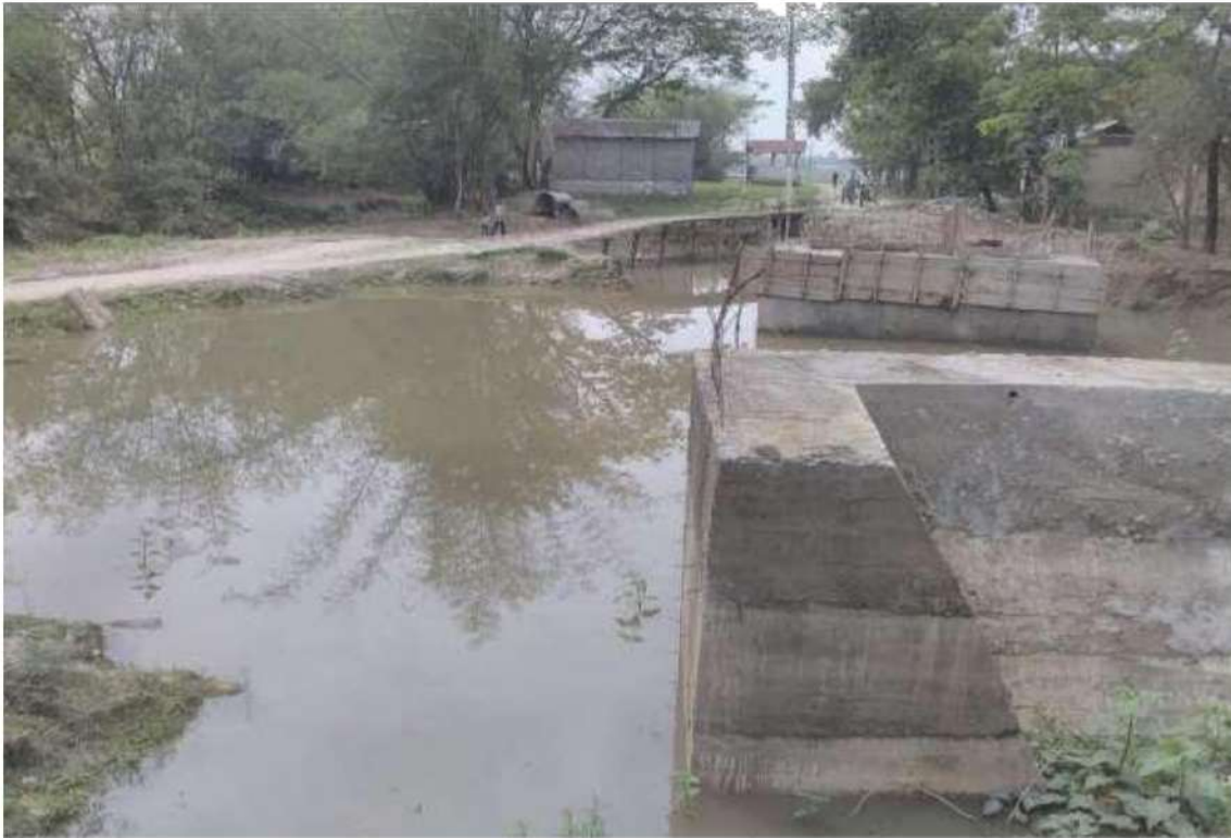
Figure 4.2 Poor conditions of the roads in Ghorbhiton-Bherbheri area
