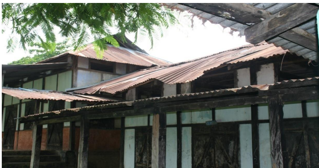
The picture shows damage due to hailstorm in school building
